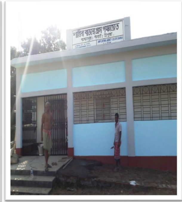
Name of Work: Const. of Panchayat Ghar GP: Shantir Bazar Block: DurgaChowmuhani District: Dhalai
