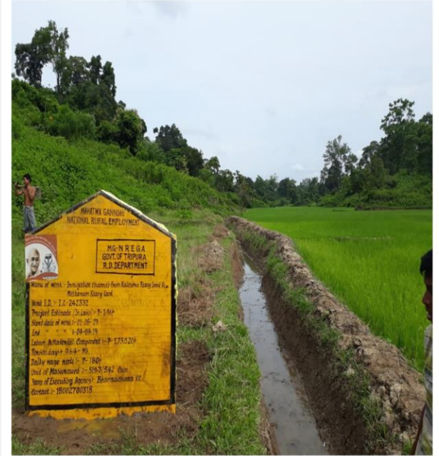
Name of Work: Irrigation Channel GP: Bhoomracherra VC Block: Amarpur District: Gomati
