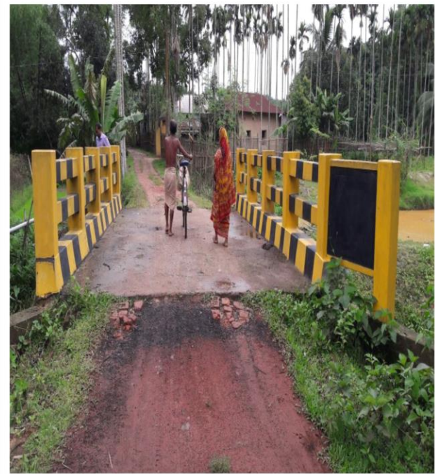
Name of Work: RCC Box Culvert GP: Kalachari Block: DurgaChowmuhani District: Dhalai
