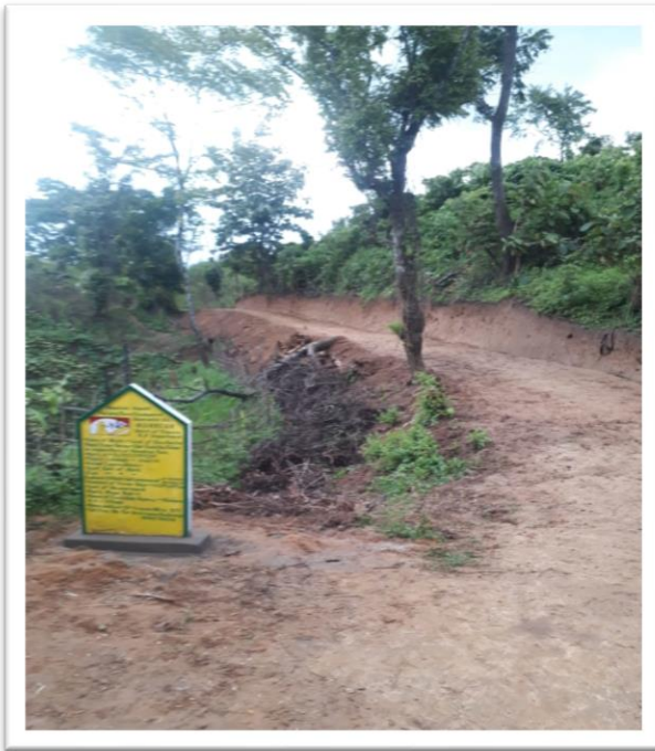
Name of Work: Formation of Road GP: Ailmara VC, Block: Shilachari District: Gomati
