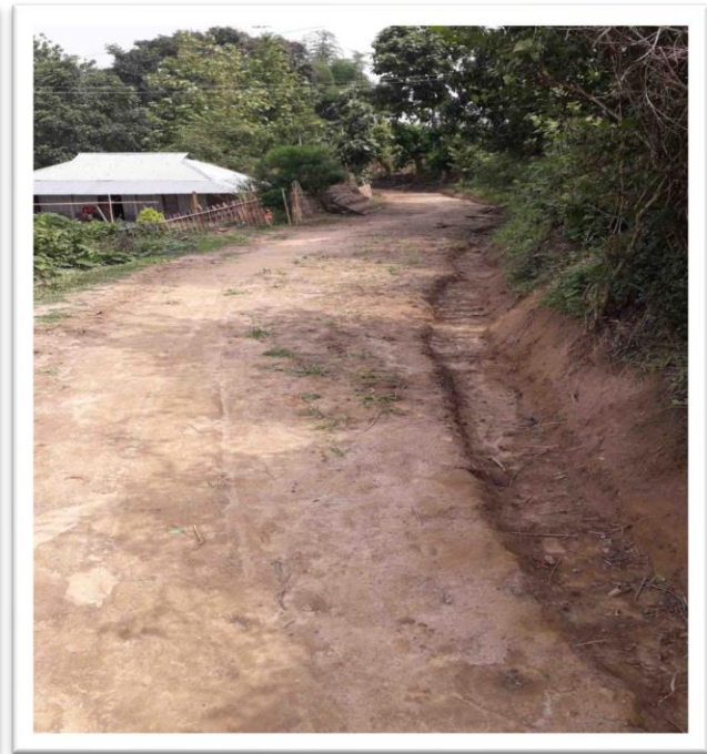
Name of Work: Formation of Road GP: South Sangang VC Block: Ompi District: Gomati
